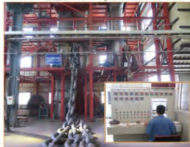
计算机控制的链链热处理炉 Heat Treatment Furnace Controlled by Computer
